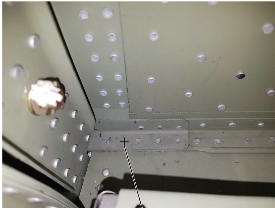
Location of possible missing rivet
